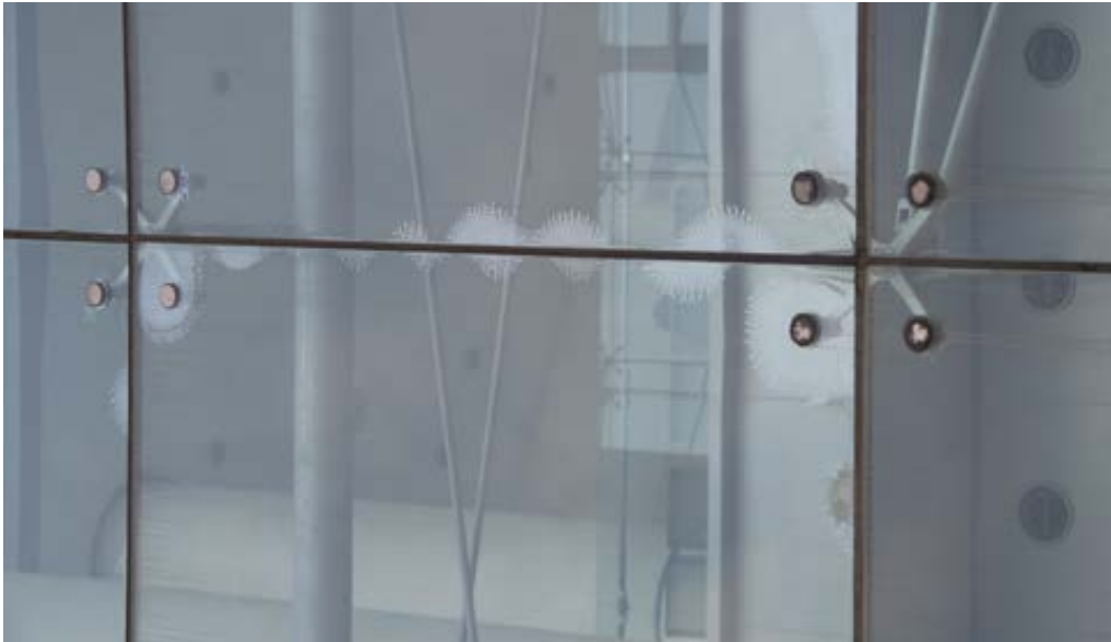
Typical defects caused by delamination.
